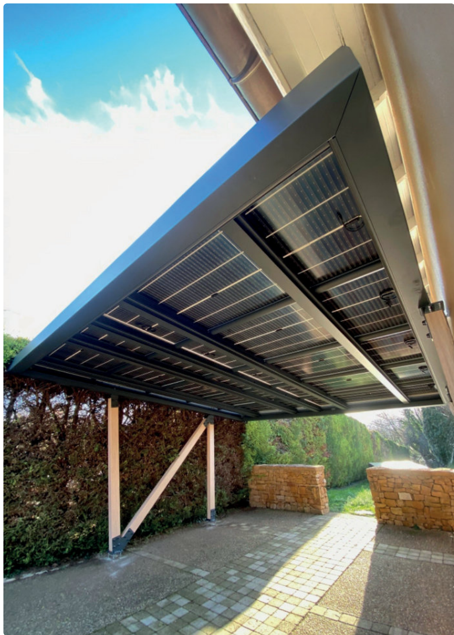
Installation 6 kWc- 2 places
